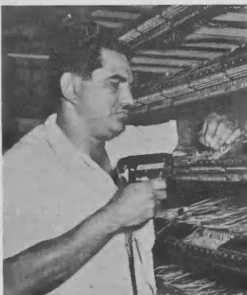
G. Arends makes crossconnection at Telephone Exchange for new personal numbering system.
